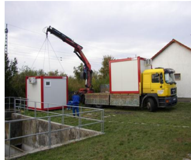
Mobile station was installed in Waste Water Treatment Plant (Várpalota)
